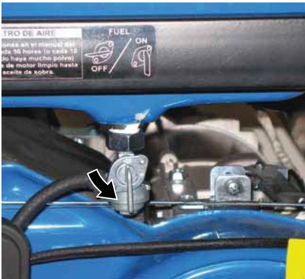
Figure 27 – Fuel Shutoff Valve in the ON Position
