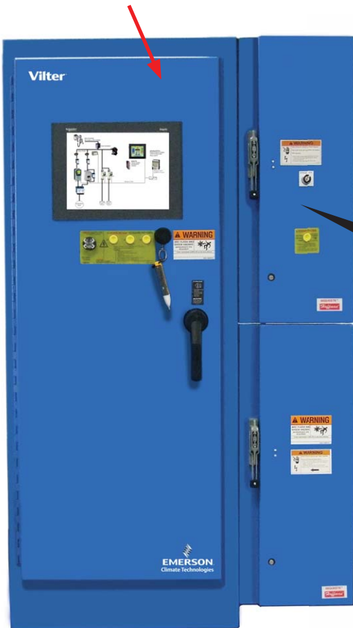
Main Motor Starter Enclosure
