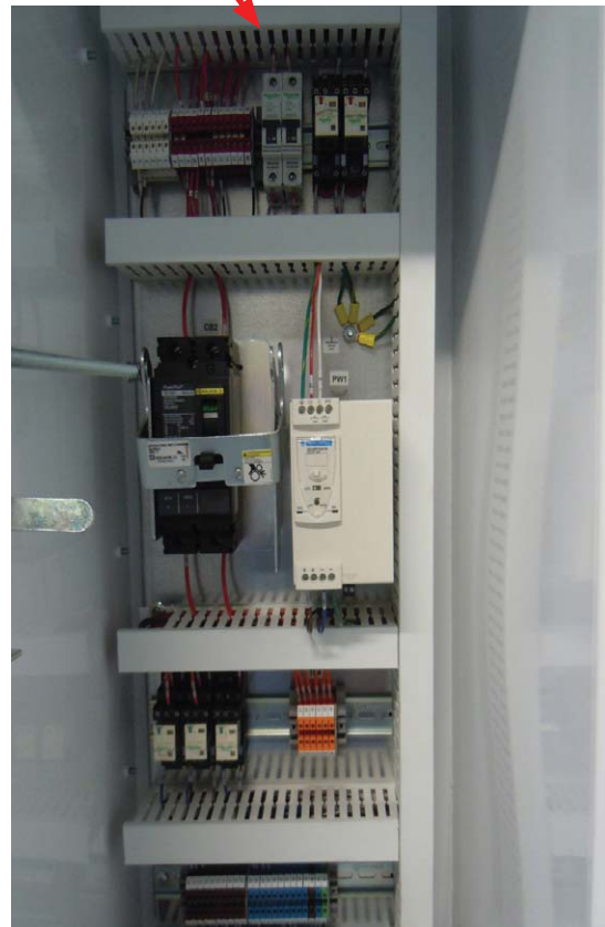
Control Circuit and Components Enclosure
