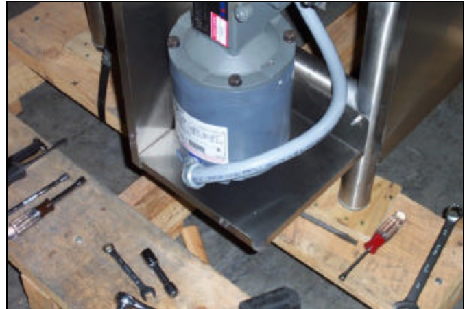
The WRONG way to mount the drive motor.
