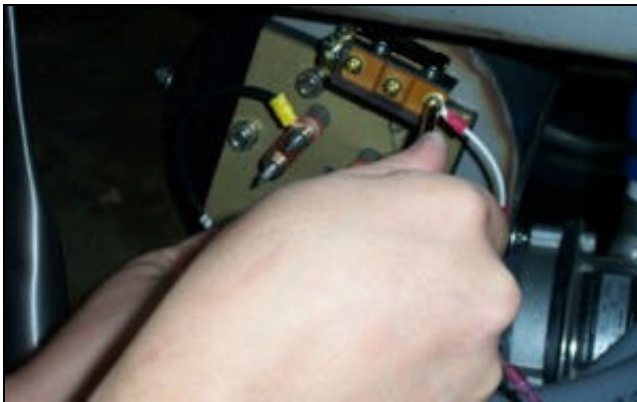
Securing jumpers to the thermostat.
