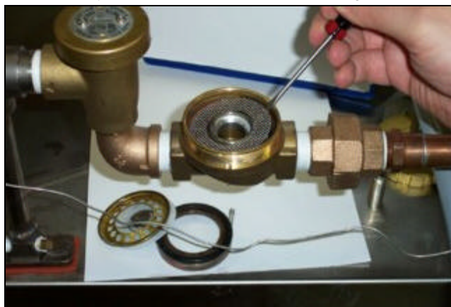
Removing the mesh strainer screen
