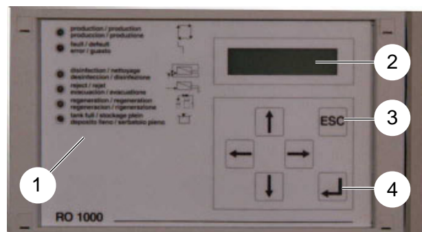
Figure 5 Control panel and display
