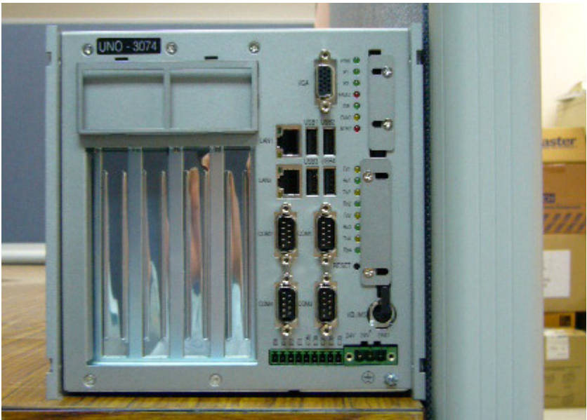
Figure 3.7: UNO-3074 Improper Installation (2)
