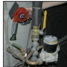
Thaw Frozen Pipes
