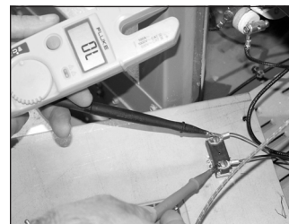
Testing the door push-button safety switch.
