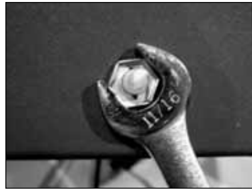
Figure 8.14 Install the speed control (rheostat). The speed control mounts to the decorative cover previously removed. Insert the stem of the speed control through the hole located on the right side of the cover. Secure with the pal nut using an 11/16 in. wrench.
