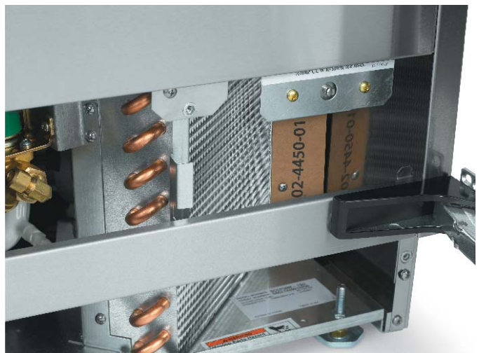
Condenser and Bin Thermostat
