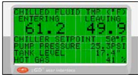
Figure 16: Main Chiller Status Screen
