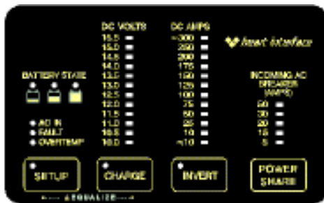
Remote Control Panel
