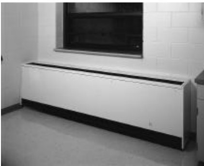
Figure 6: Typical classroom unit ventilator installation
