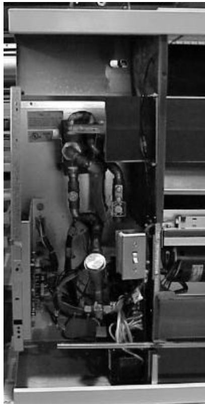
Figure 10: Horizontal classroom unit ventilator end pocket
