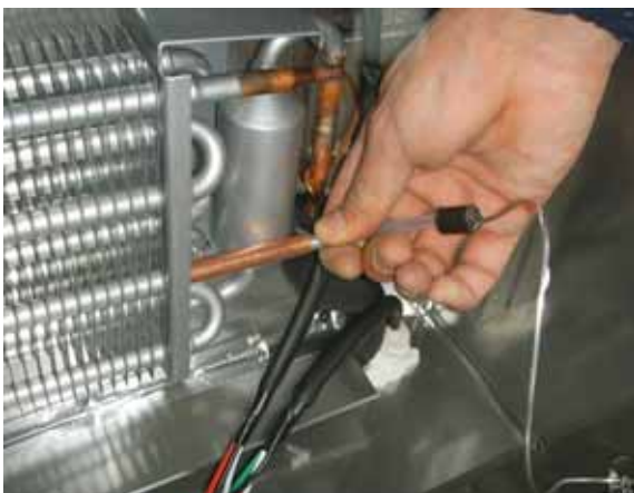
TEMPERATURE CONTROL & EVAPORATOR
