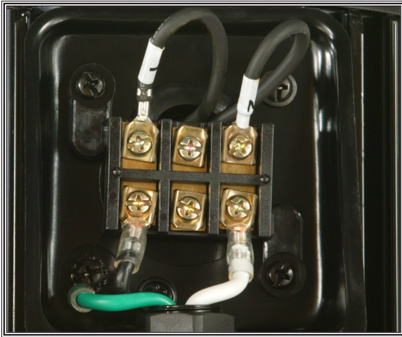
Figure 58. W1808 motor wiring.
