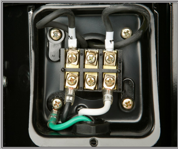
Figure 61. W1809 motor wiring.
