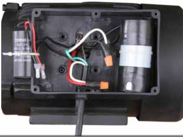
Motor Junction Box
