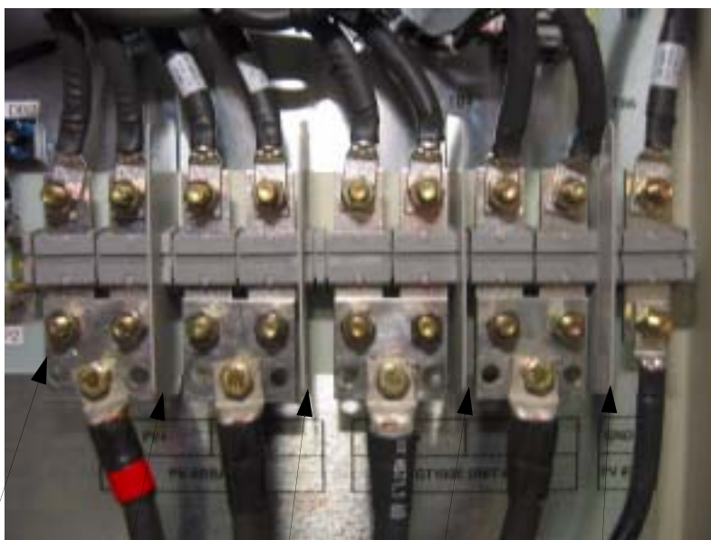
Combiner Box PV ARRAY #2 PV (+) Terminal Combiner Box PV ARRAY #2 PV (-) Terminal Combiner Box GT100E #2 PV (+) Terminal Combiner Box GT100E #2 PV (-) Terminal Combiner Box PV ARRAY #2 GND Terminal
