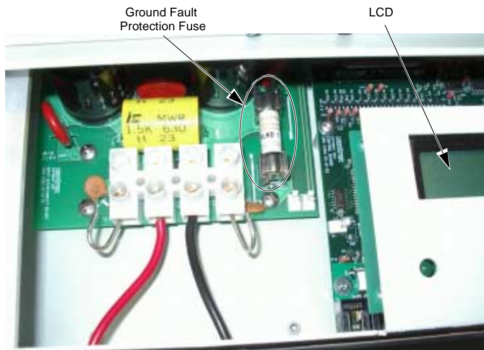
Figure 6-1 Location of Fuse, Front Panel Cover Removed
