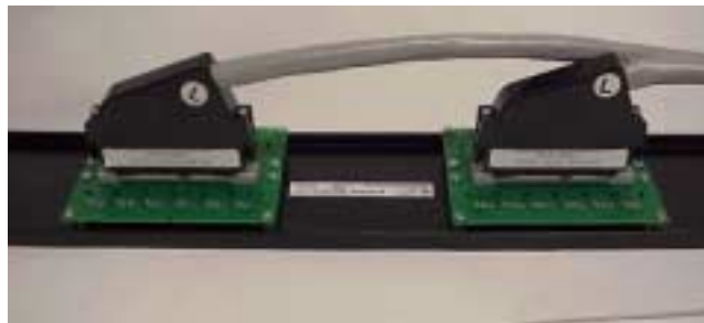
Figure D-2 Cable Attached to the Panel
