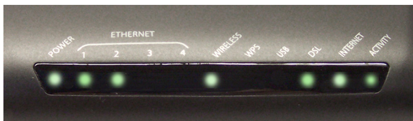
LEDS SHOWING NORMAL OPERATION
