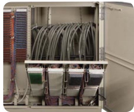
NCX-1000 shown with drop down panel opened for easy access to OSP cable stubs for splicing into DSLAMs and network.
