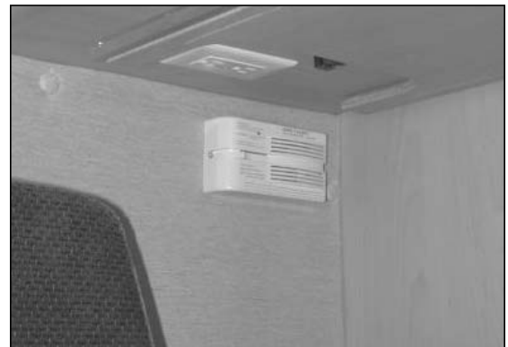
Picture F-P2: Carbon monoxide leak detector.
