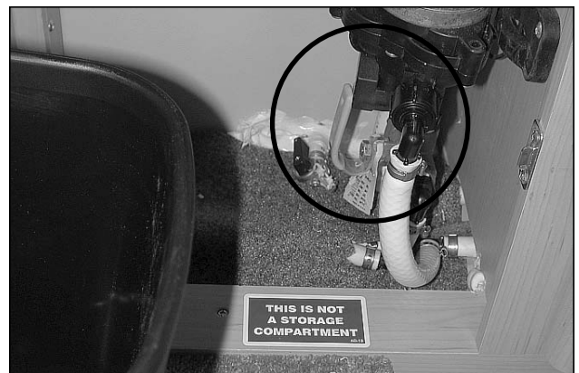
Picture G-P2: Selector valve position for supply from the exterior fresh water tank.
