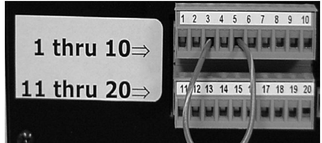
Figure 16. 12 Volt Supply Jumper
