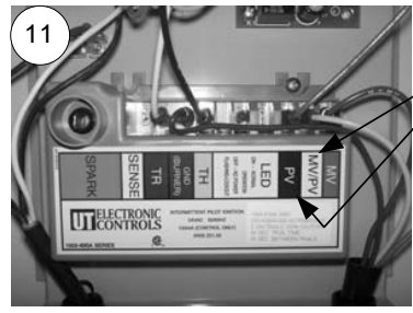
Check across "MV/PV" & "PV" terminals
