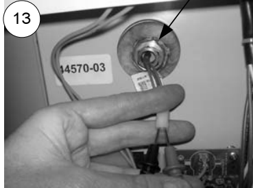
Check across RED wire leads of lower thermister (ECO).
