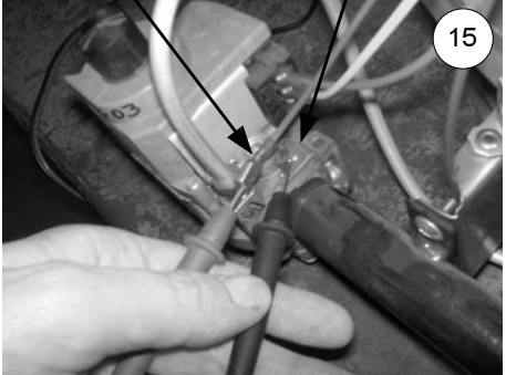
Checking main valve (MV) voltage to gas valve.
