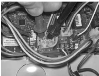
Checking MV pin terminal to gas valve wire harness for 24 volts output to gas valve during heating cycle (pilot must be lit with no sparking).
