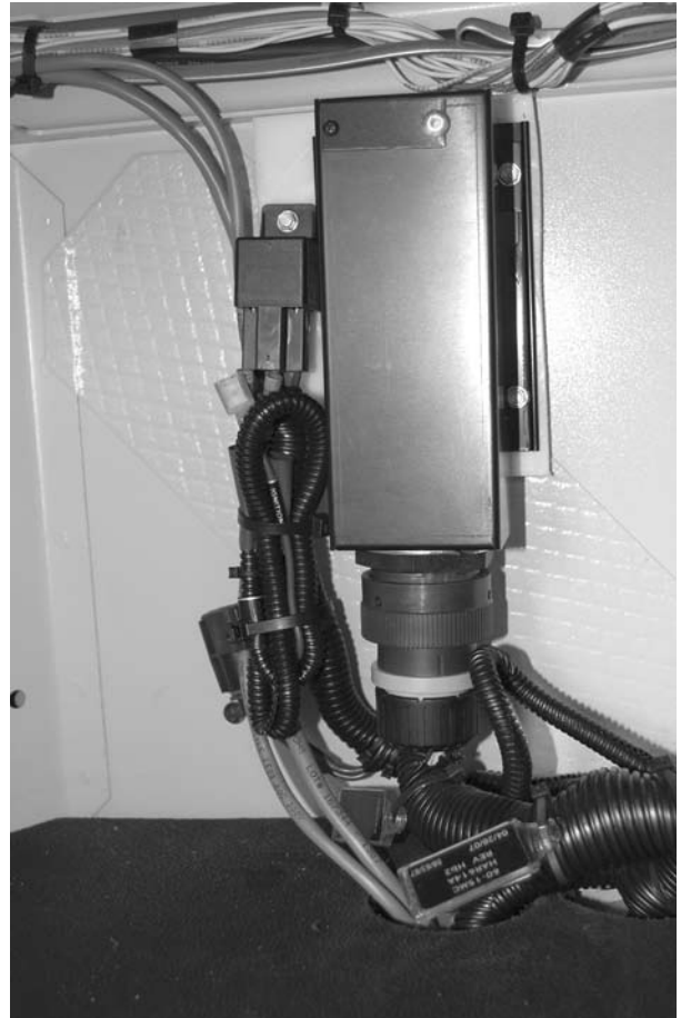
Figure 7 – Regulator mounted inside truck
