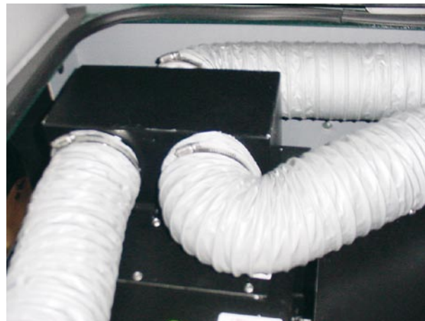
Figure 19 - CHEB with ductwork installed
