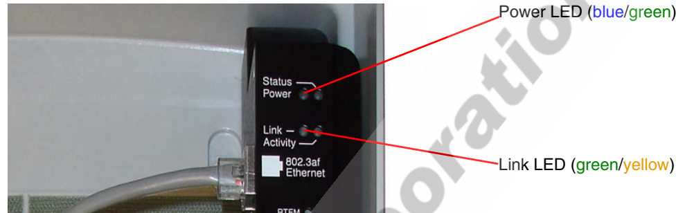
Figure 2-5. Loudspeaker Amplifier LEDs—Power and Link
