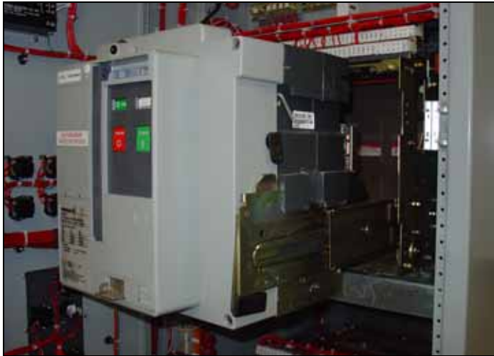
Figure 26. Switching Device Drawn Out from the Transfer Switch.
