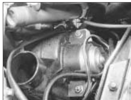
9C.85 Fuel injector cooling fan
