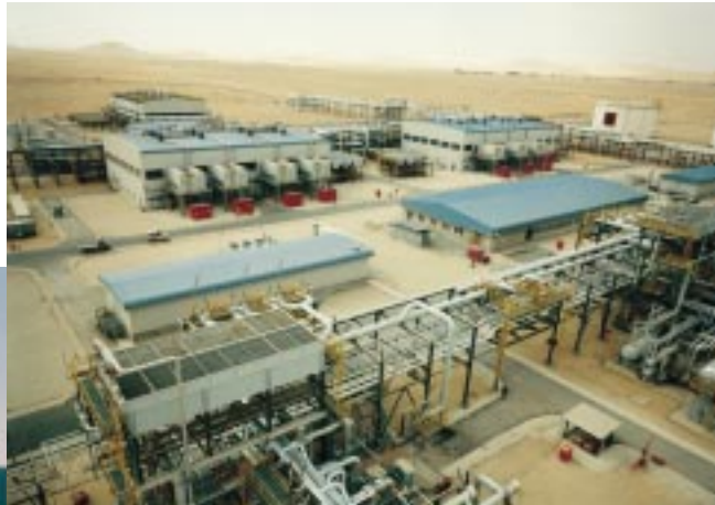
Mesaieed - Qatar MS5001 Turbogenerator units for Fertilizer plant
