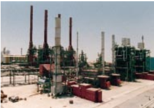
Rhourde Nous - Algeria MS5001 - MS3001 Gas Turbines and 2BCL 406B Compressors
