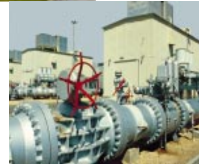
Sbikha - Tunisia PGT 25 - PCL603 Pipeline Compressors
