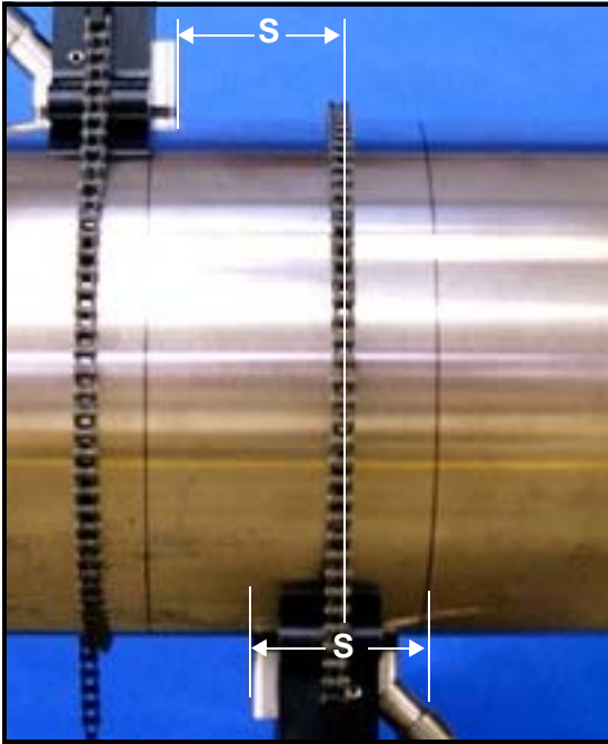
Figure 3-21: The Installed CFG-PI Fixture, with Calculated Spacing
