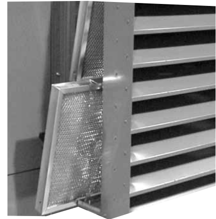
Outdoor air intake hood mesh filter access
