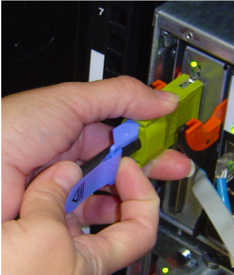
Figure 2-1: Connecting InfiniBand Cables
