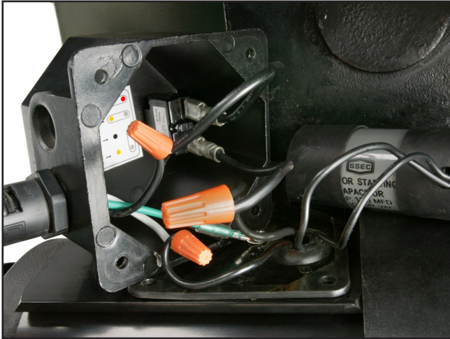
Figure 61. Motor junction box wiring.
