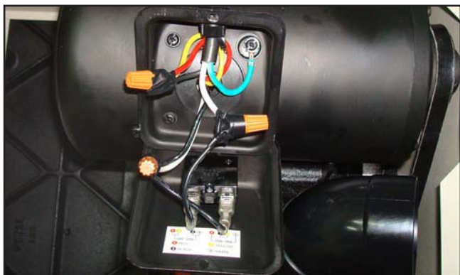
MOTOR JUNCTION BOX
