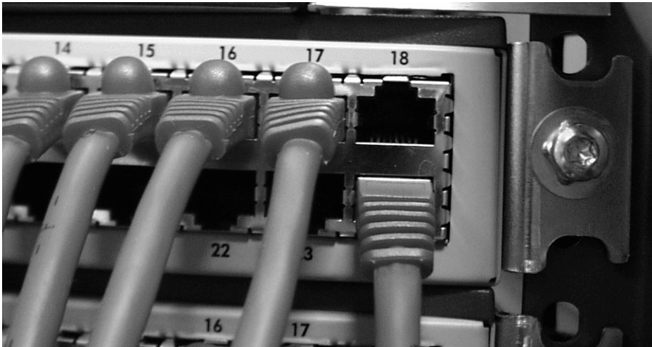
Figure 2-13 Connecting HP ProCurve Hub to LAN
