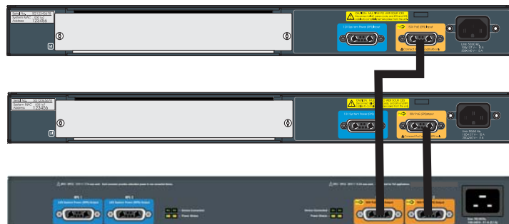
Figure 2-14. Connecting EPS to 2, 24 port switches.
